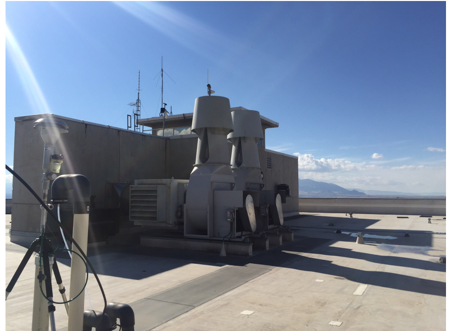
The Penthouse. Also, notice the exhaust vents from fume hoods...
